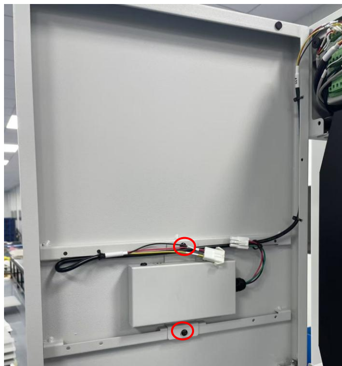
Figure 137. LED Light Module Removal
